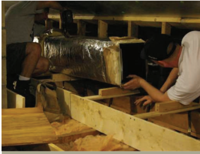
FIGURE I-13 Duct insulation increases system energy efficiency.
